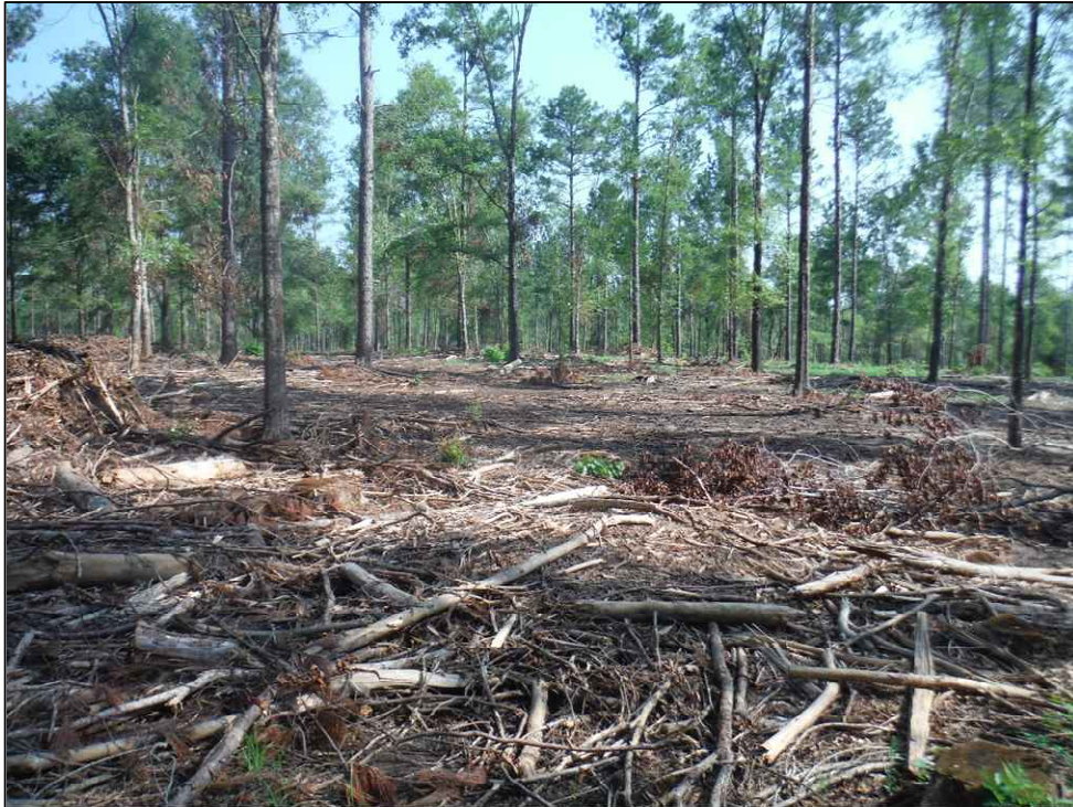
Figure 2.3. Portion of the project area that has been cleared of vegetation, facing north.
