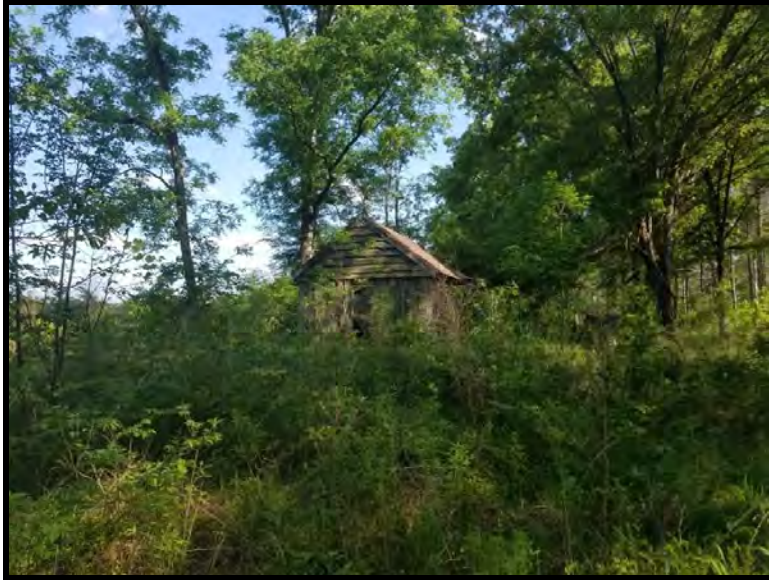
13 View of the rear of a former barn/shed located on the western portion of the Property.
