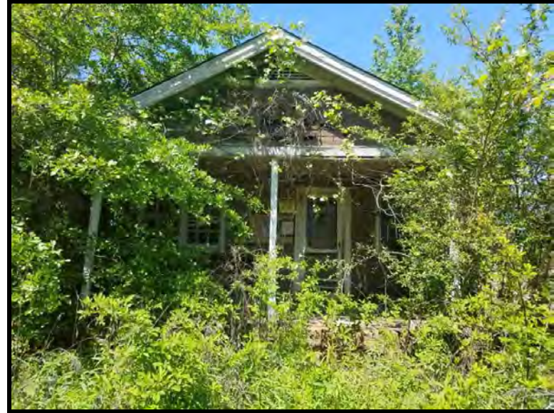
10 Residence located on the north-central portion of the Property. Currently used as a hunt club cabin.
